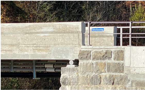
Engineering the existing means knowing how to respect the existing: focused and precise examination of reinforced concrete, steel roller bearing, and natural stone masonry abutment from 1935 was the key to non-invasive intervention to extend the service duration, thereby avoiding demolition. Photograph by the author
