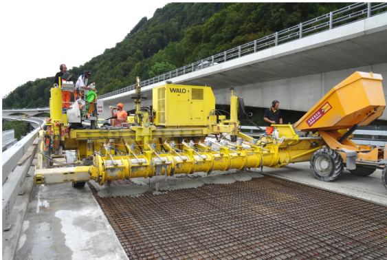
This 2.1-kilometer-long highway viaduct, built in 1969, was rehabilitated and strengthened in 2014–15 by means of the new UHPFRC (Ultra-High Performance Fiber-Reinforced Cementitious composite material) Technology (developed at EPFL). The realized project was cost-effective and did not impair the appearance of the viaduct which is a monument of national value. Photograph by the author
