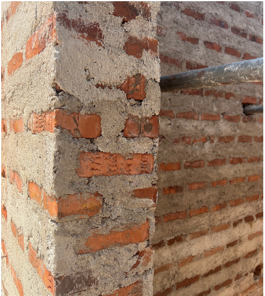
A construction site in Sri-Lanka, 2024, somewhere by the sea. Photographer: Jo Taillieu Architecten
